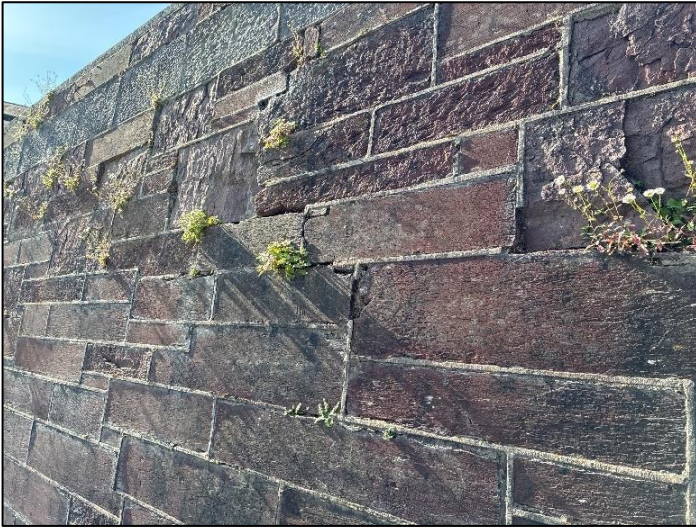
Figure 4-3 – Stone wall (BL1) with vegetation including maidenhair spleenwort ( Asplenium trichomanes ) and daisy ( Bellis perennis ) on Abbey Street.
